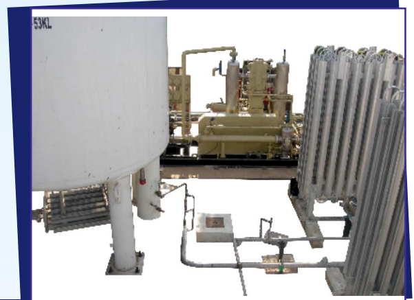
S.S. Piping Instrumentation
